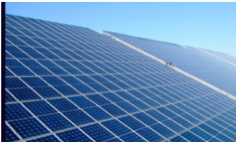
Solar Panels at Winery
